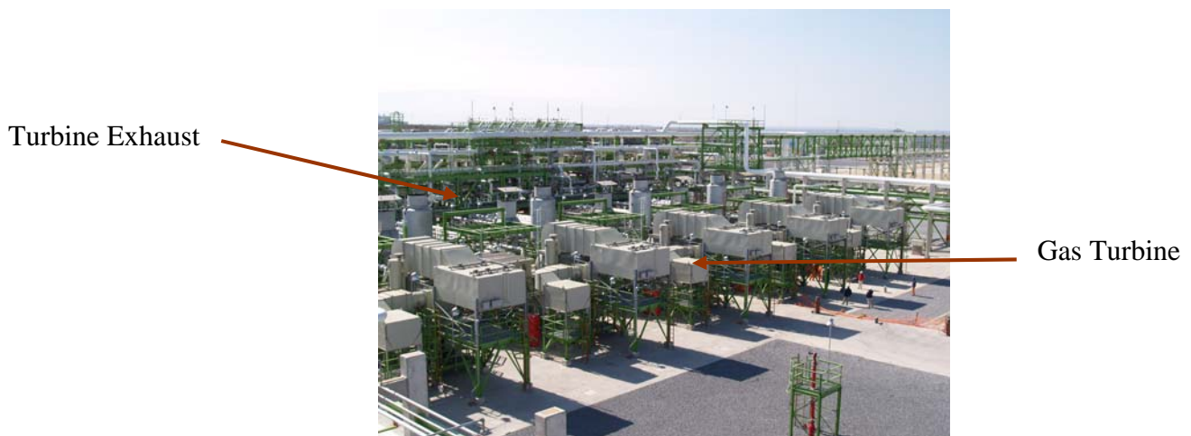
Figure 3 – Waste Heat Recovery Units on Gas Turbine Exhaust
