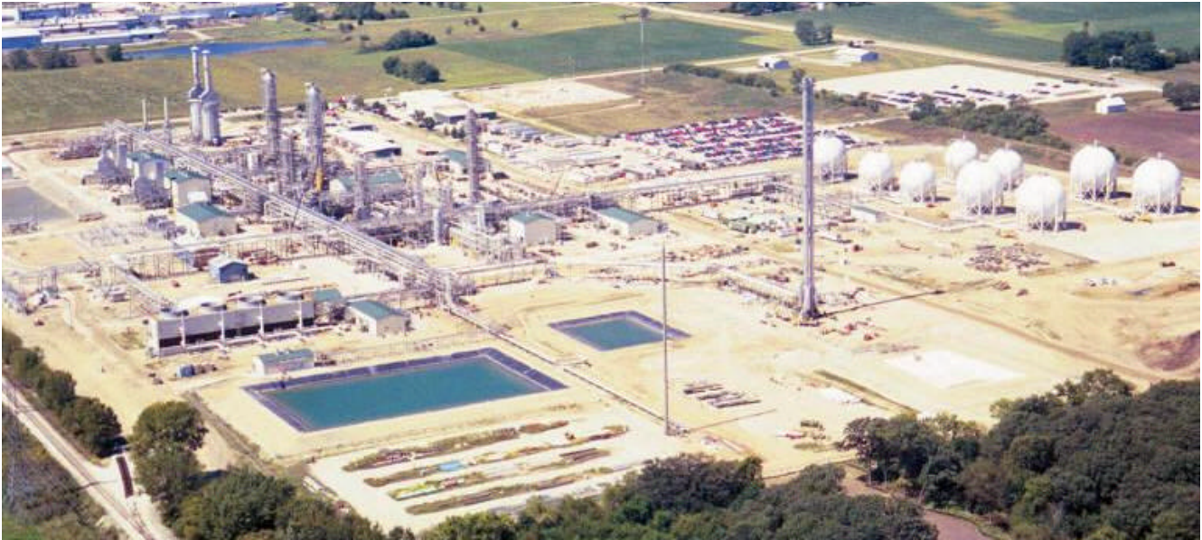
Figure 2 – Aux Sable NGL Recovery Plant
