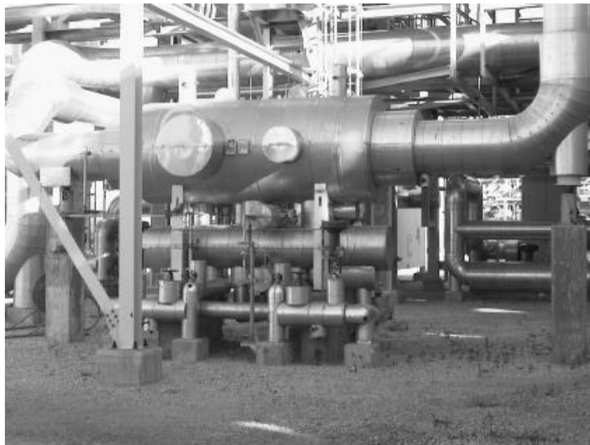
Figure 5 – Aux Sable Cold Separator
