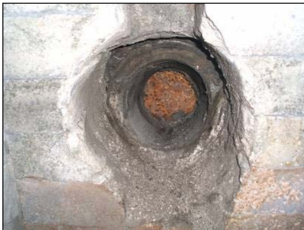
Figure 6. Acid Gas Bypass Nozzle Failure
