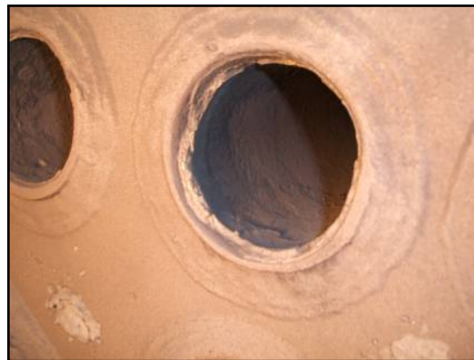
Figure 11. WHB Tubesheet Joint After 25 Years Service
